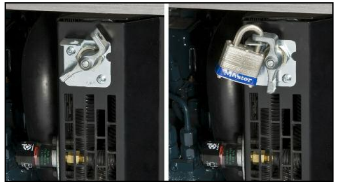
Battery Ignition Disable Switch for Lock Out/Tag Out
